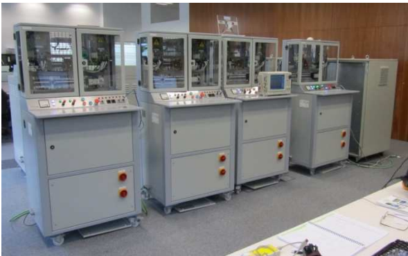
Fig. 2 Four cabinets of the microgrid.
